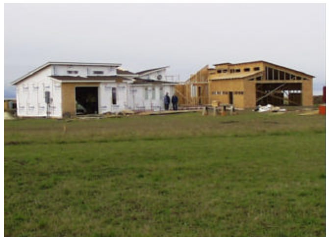
Pat Schoen and Connie Engvall are building their home at the west end of Greywolf Road.
